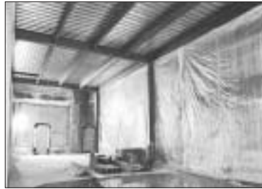
photo--Michael K. Wilkinson--The InTowner. Shown here is the interior construction underway on future retail spaces inside the Tivoli Theater building, as reported in the accompanying "Project Up-dates" article at page 1.
